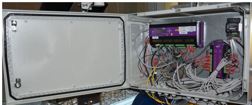
Figure 3.14: Data logger DT85 and channel extension module CEM20 setup in watertight box from a different angle.
