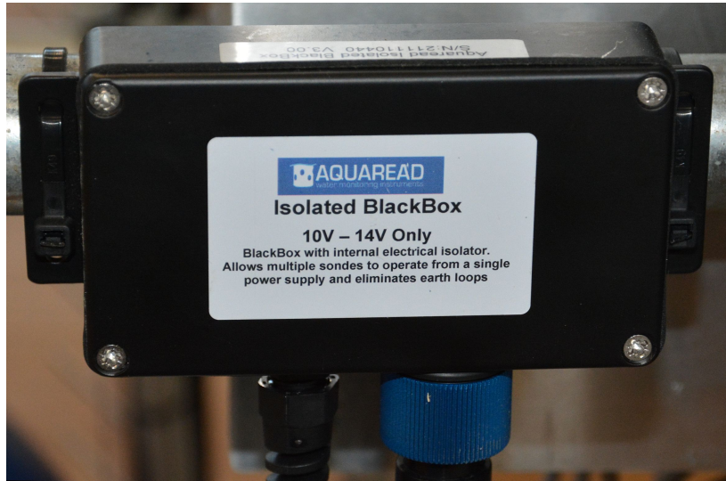
Figure 3.29: Aquaread black box connecting the aquaread probe (AP-7000 / AP-5000) to the datalogger DT85. The aquaread black box acts as signal converter, making the signal readable for the datalogger.
