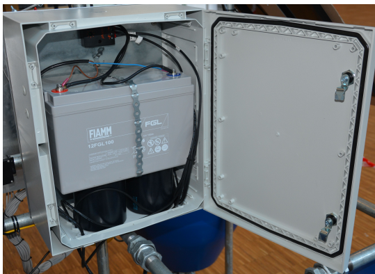
Figure 3.8: Watertight battery box containing the battery and charge regulator.
